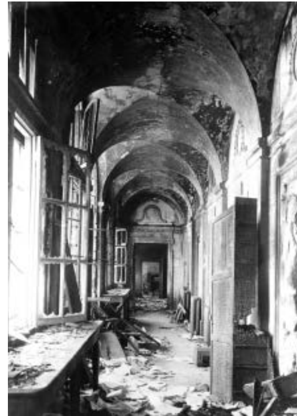
Custom House, interior corridor after fire, June 1921 IAA Photographic Collections, 9/63Y15
